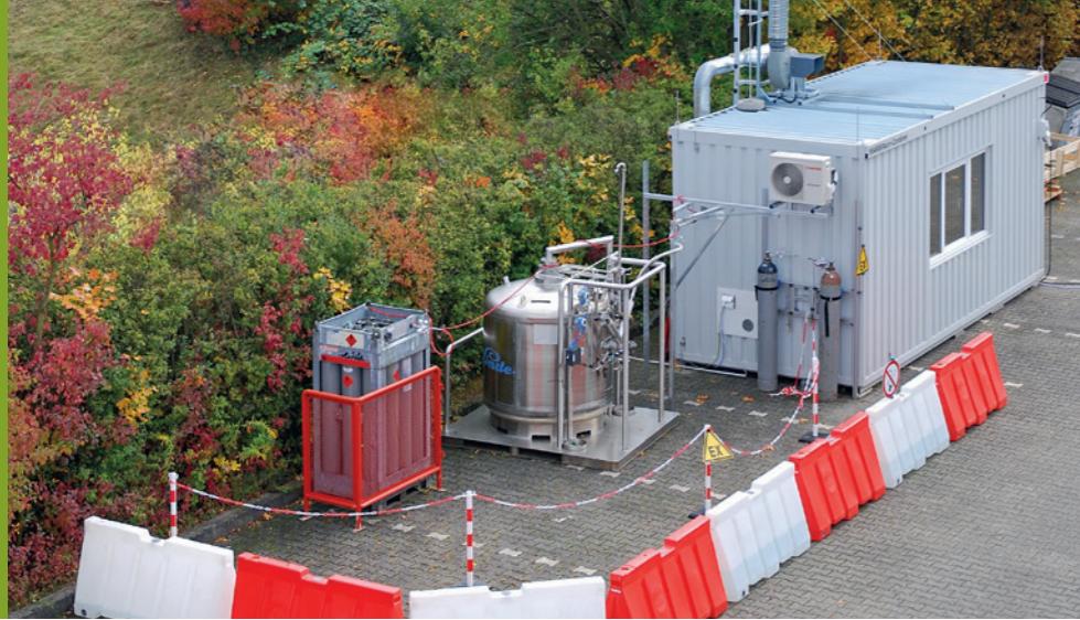
Test plant for cryogenic fuels (in an external container)
