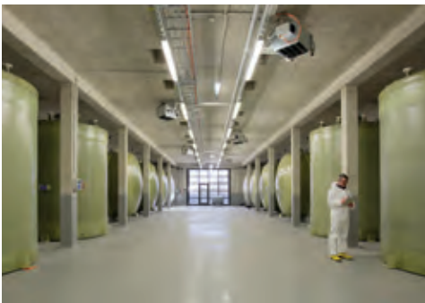
Tanks der Redox-Flow-Batterie am Fraunhofer ICT
